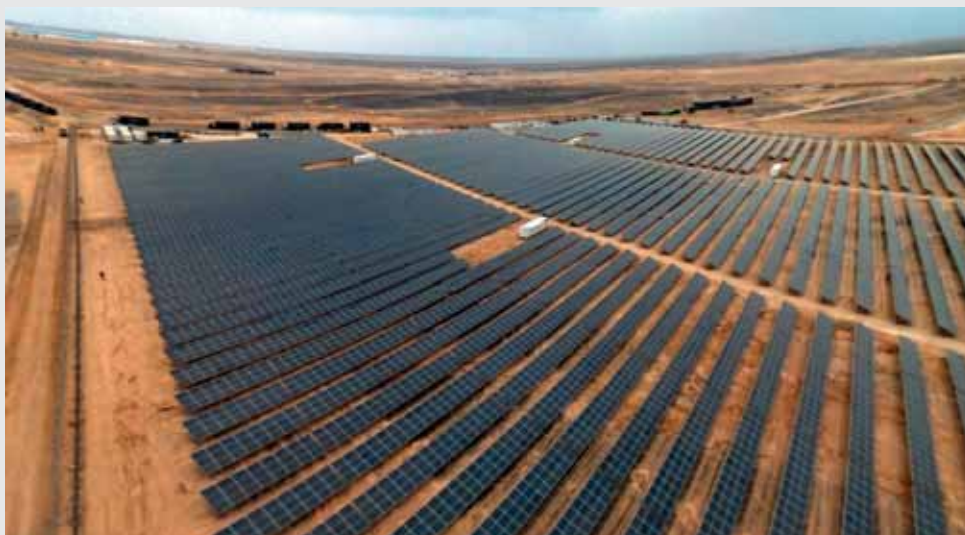
Arabia One Solar in Jordan took an integrated approach to O&M planning
