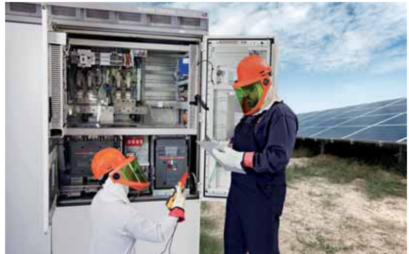
Credit: SMA Solar
