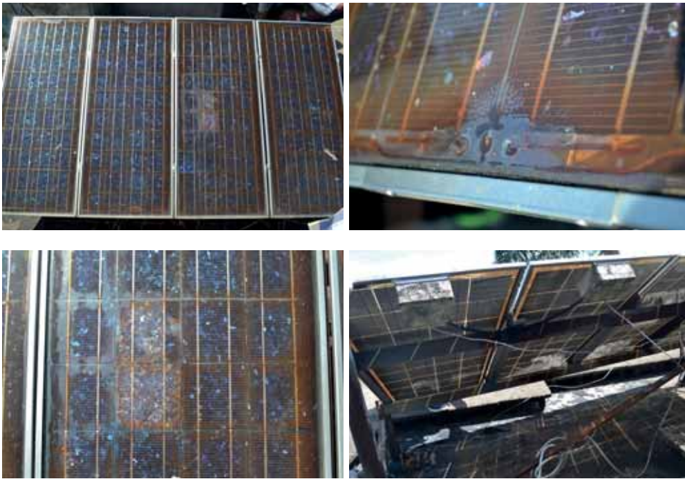
Figure 5. A fifteen-year-old (installed for 19 years) double-glass module in Hainan, showing cell corrosion and encapsulant yellowing
