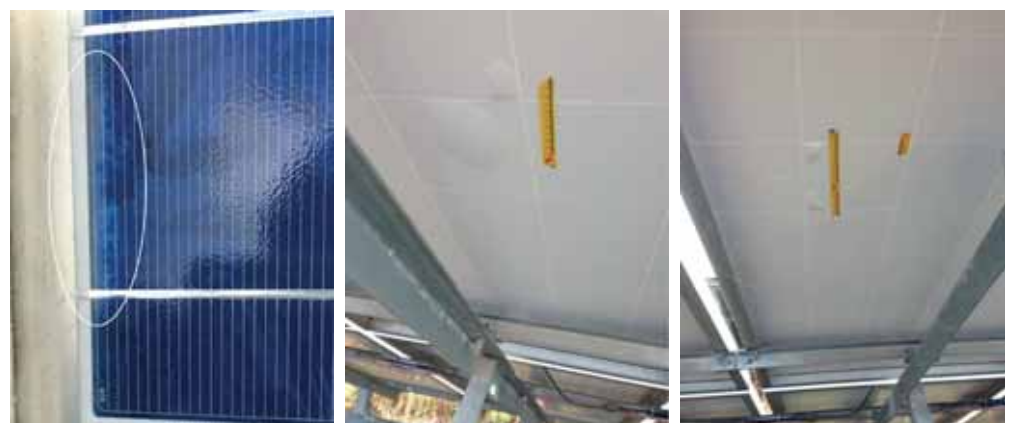
Figure 6. Four-year-old field module in Jiangsu: (a) moisture ingress issue; (b–c) PVDF backsheet inner layer bubble/delamination issues
