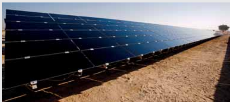
The 13MW first phase of the Mohammed bin Rashid Al Maktoum Solar Park.
