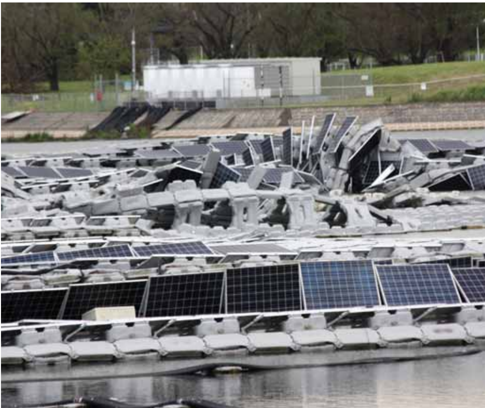
Figure 5 Typhoon caused fire on Japan's largest floating PV site on Yamakura Dam in 2019
