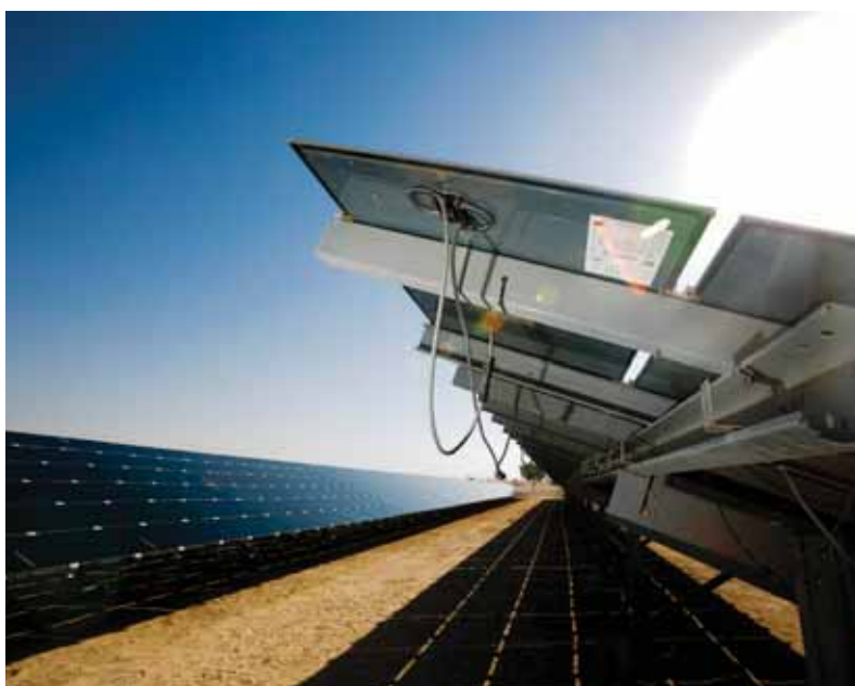
Phase 1 of the Mohammed bin Rashid solar park, completed in 2013. Image: DEWA.
