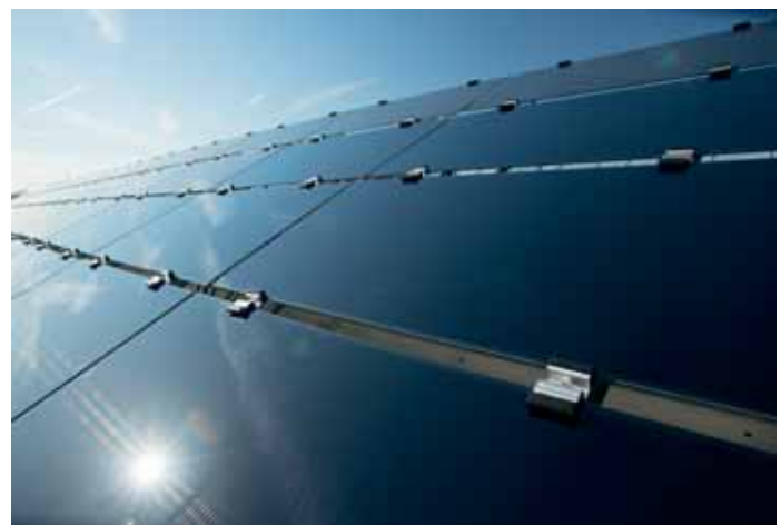
Credit: First Solar
