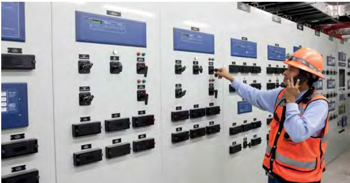
Credit: First Solar
