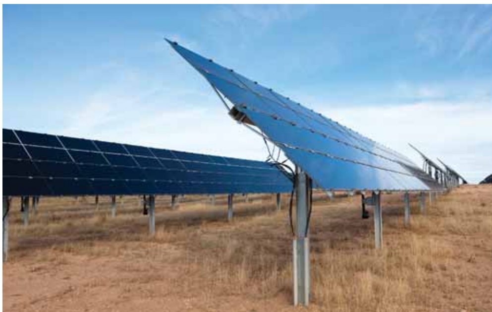
Credit: First Solar
