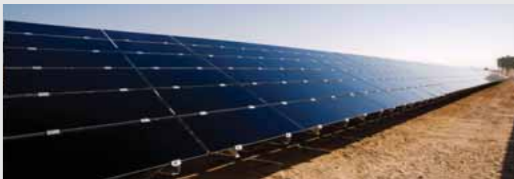
Credit: First Solar
