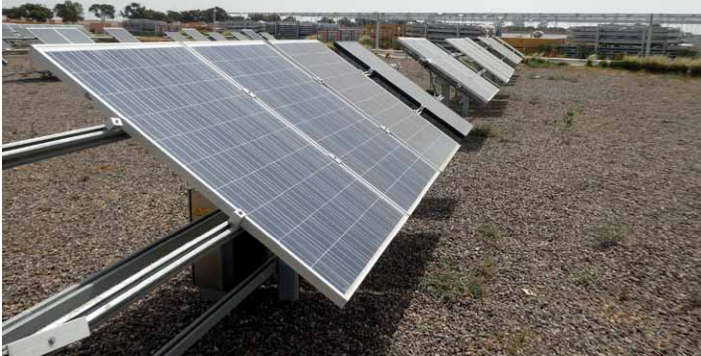
Picture 1. Outdoor measuring set-up and installed PV modules in Green Energy Park of IRESEN, Ben Guerir, Morocco [8]
