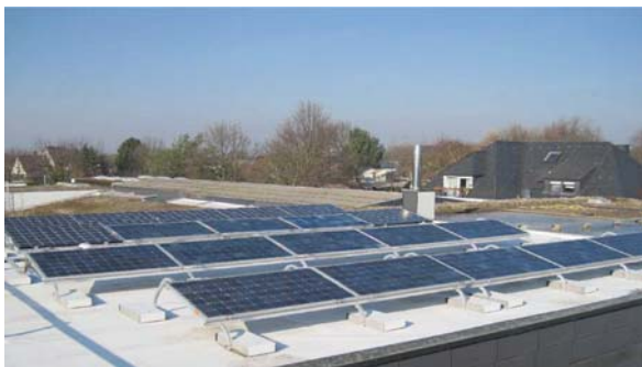
Figure 10. Rooftop test field in Geilenkirchen
