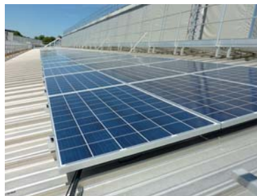
Flat-to-roof system on South/East/West pitches
