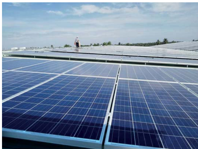
KEHUA's industrial rooftop project for a factory in Bangkok, Thailand
