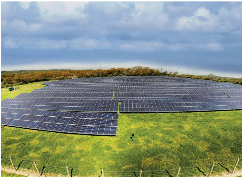
Credit: Wight Community Energy
