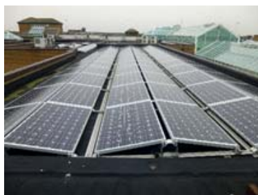
East/West facing system on flat roof
