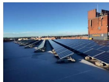
South facing system on flat roof
